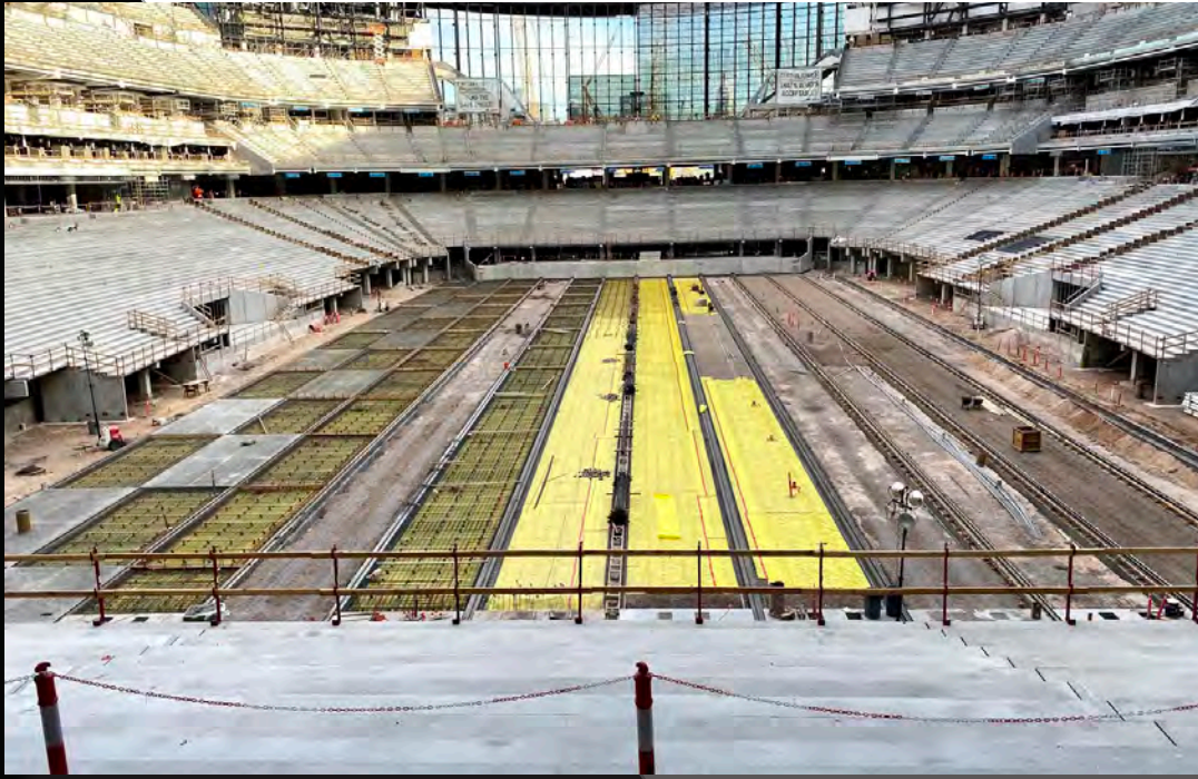
Above: View of the bowl looking north from the 100 level. Slab on grade began in January.
